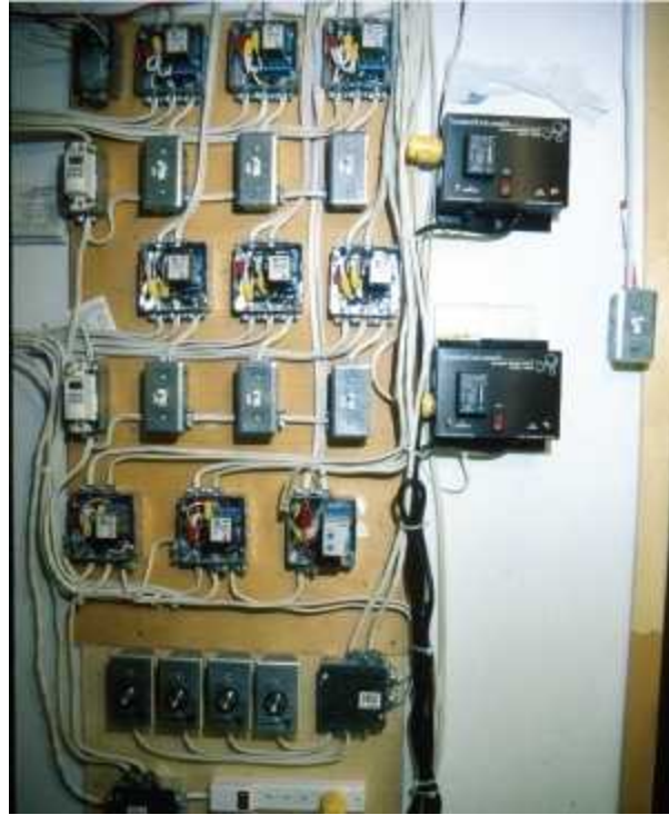
Fixing all wiring and electric devices to a control panel makes control and troubleshooting easy.
