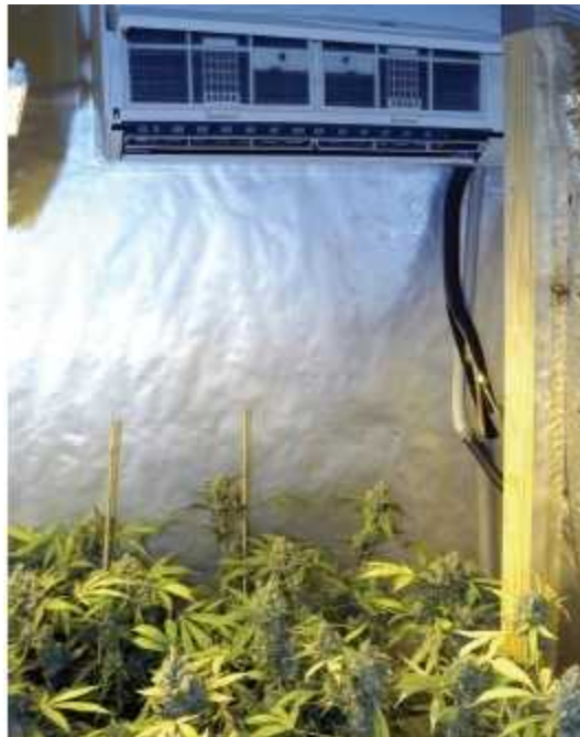
This air conditioner lowers grow room temperature and humidity. The hot radiator is outside, about 10 feet (3 m) away.
