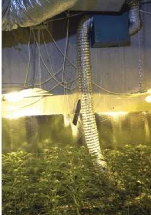
A booster fan in the gray box pushes intake air down the duct to the bottom of the garden.
