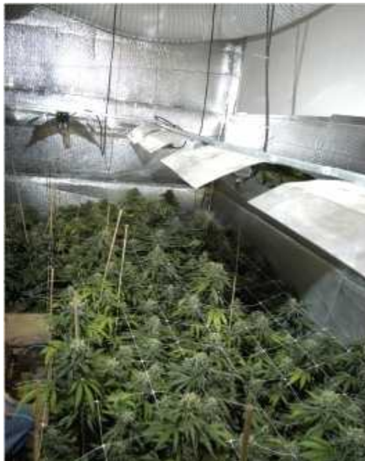
Avoid long, unnecessary ducting such as shown above. Keep ducting as short as possible.
