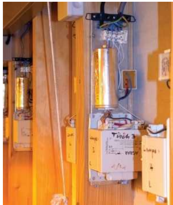
Attach ballasts to the wall so they are out of the way in the garden.
